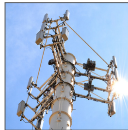
Cellular Base Station
